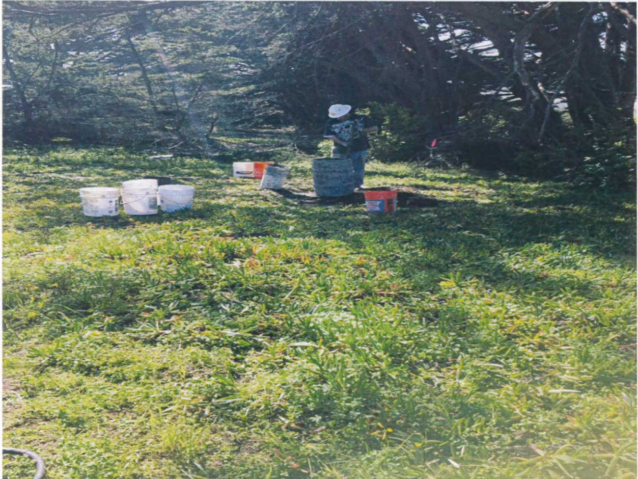
Collection of spoils and mixing of grout at test bore hole B1
