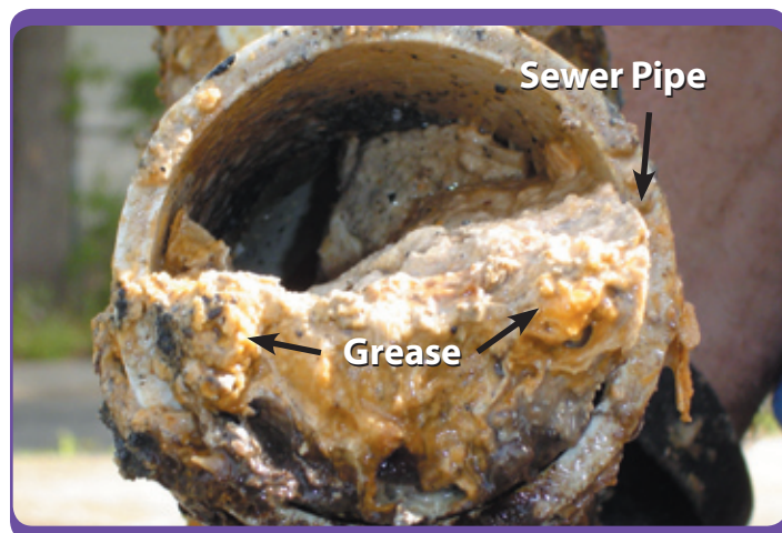
Image #3 – Grease inside of sewer pipe
