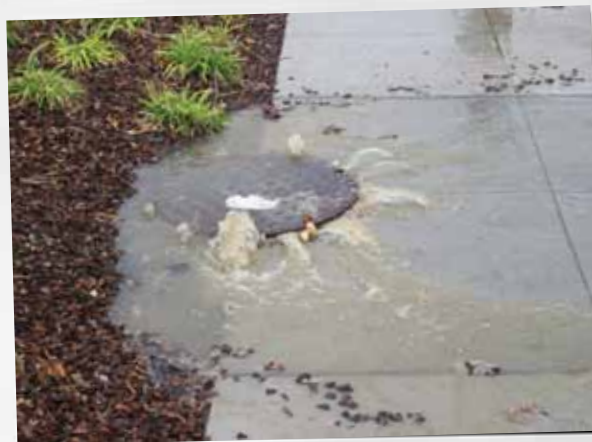
sewer overflow due to infiltration
