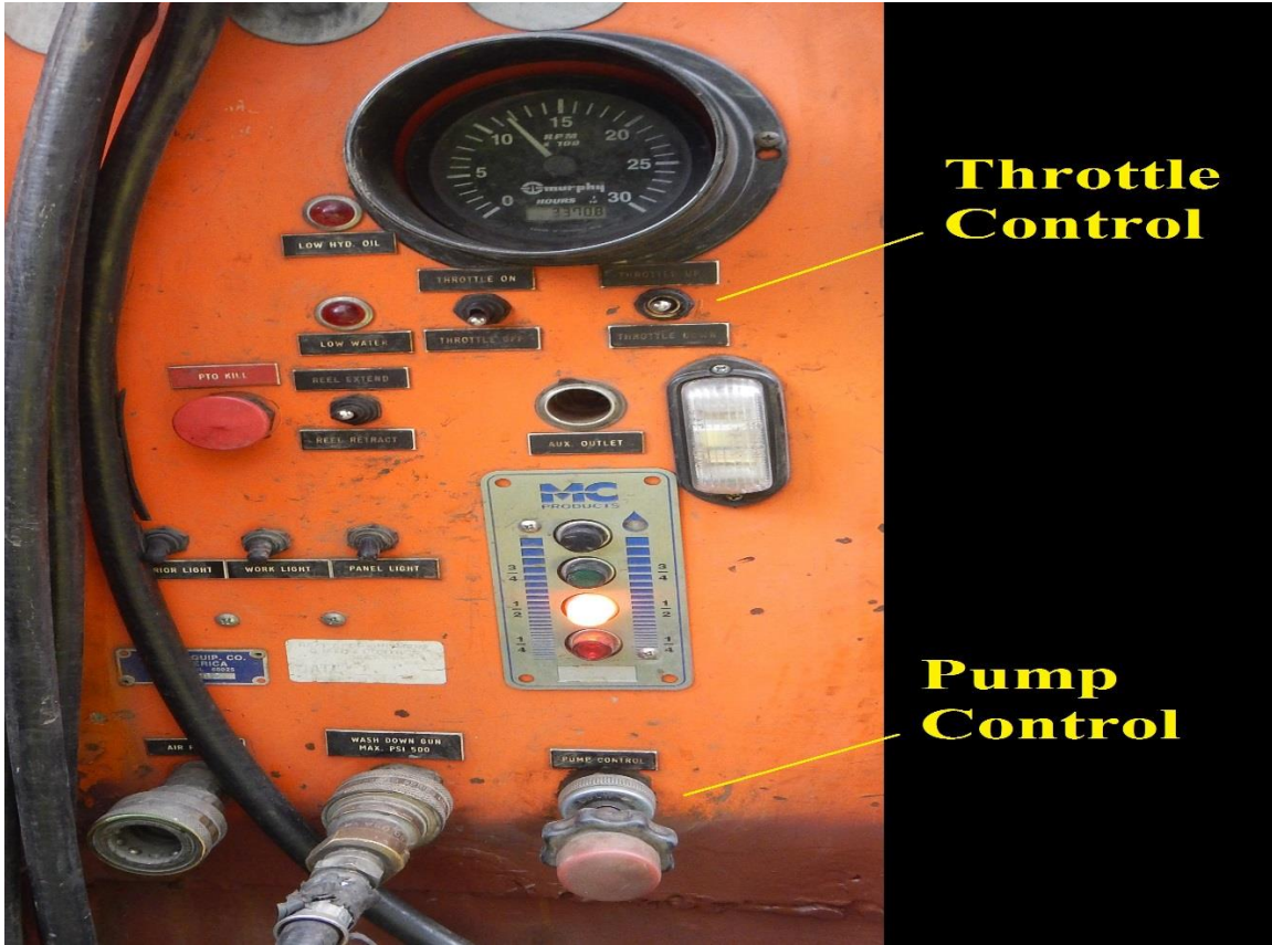
Figure 8. Rodder Pump Control Panel (572W truck)
