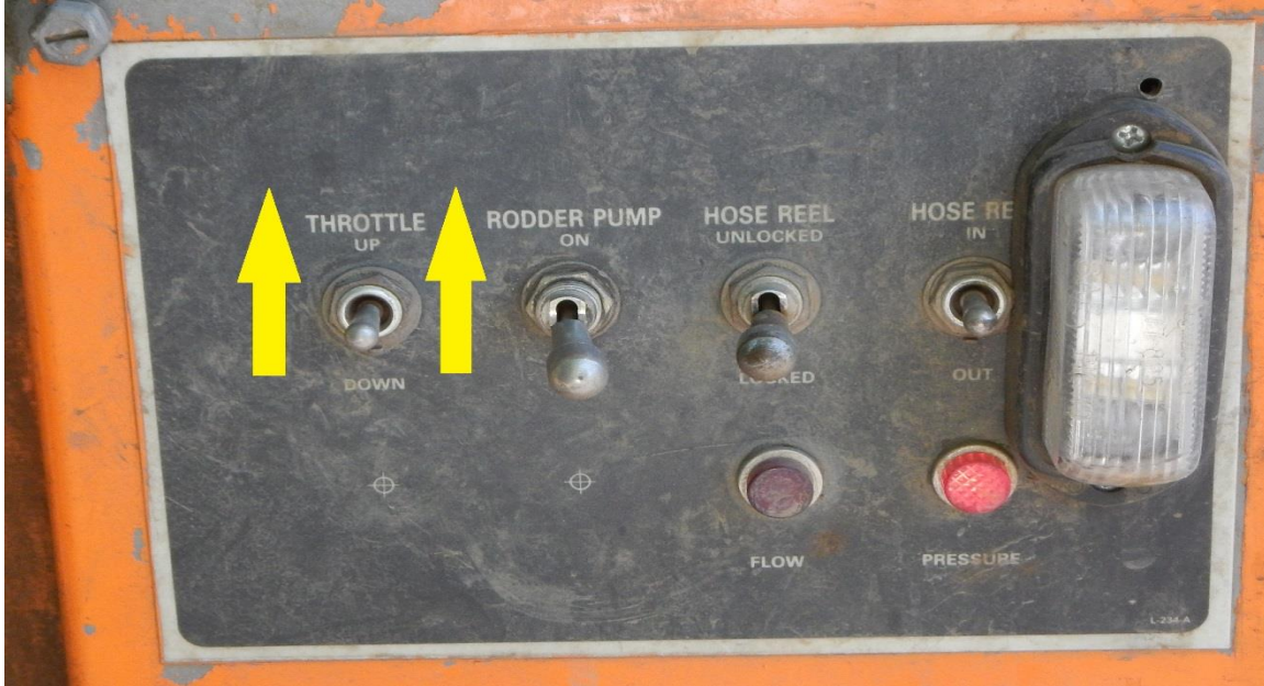
Figure 4. Rodder Pump Control Panel (513N truck)
