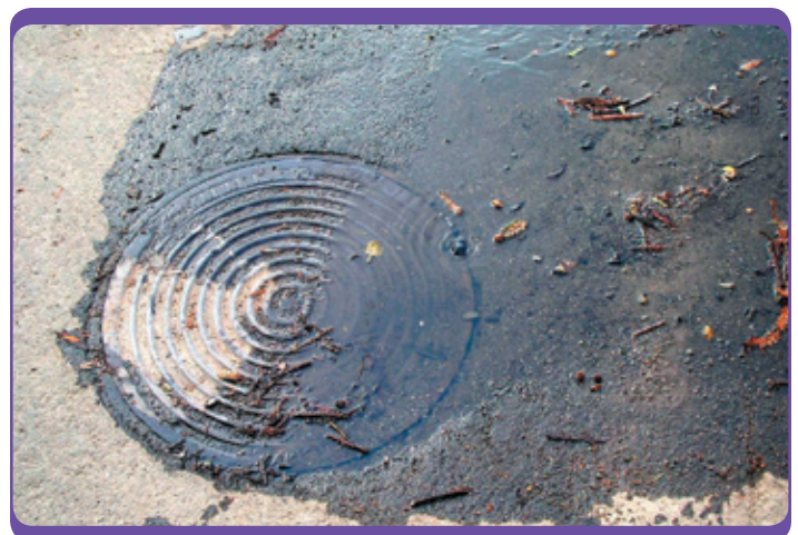
Image #10 – Sewer overflow at sewer manhole
