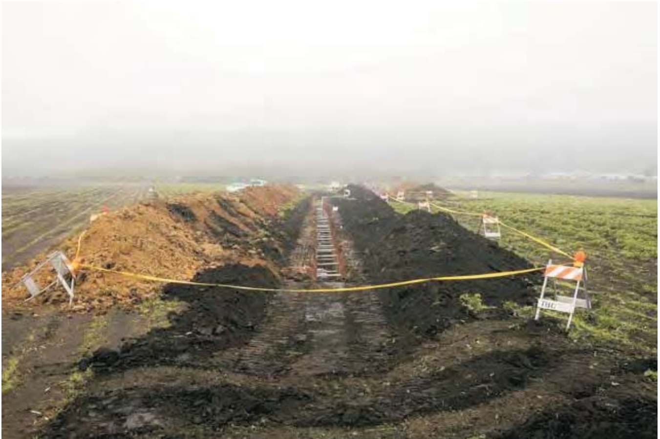
Overall View, from West End of Trench A. Note Trench B in Background, to Right
