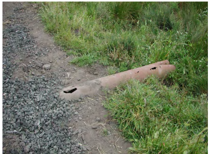
MP 43: Rusted culvert at wet area
