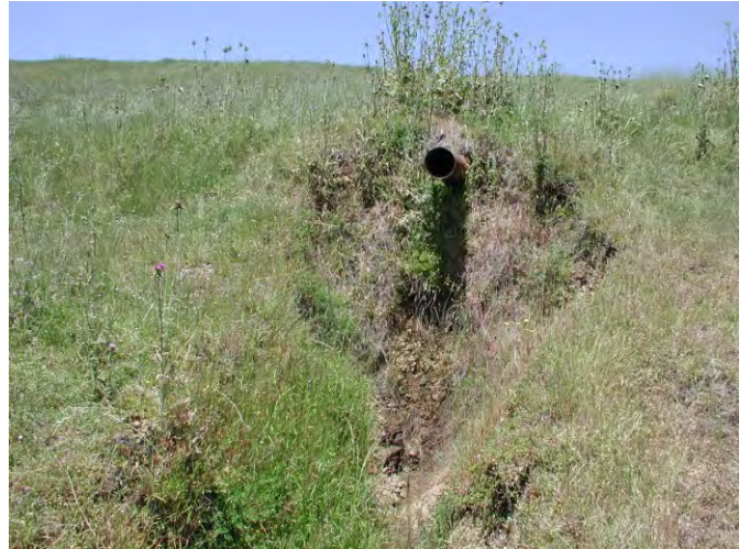
MP 32: Gully at outlet of ditch relief culvert
