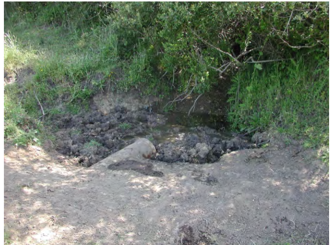
MP 48: 12" ditch relief culvert intercepting ditch flow and
