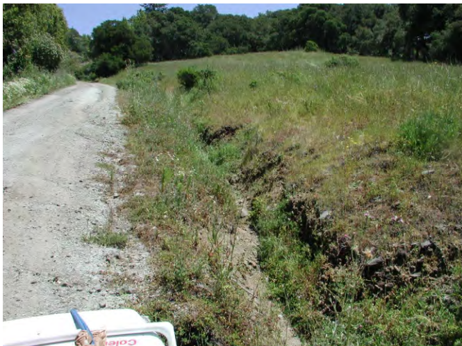
MP 11: Long eroding inboard ditch
