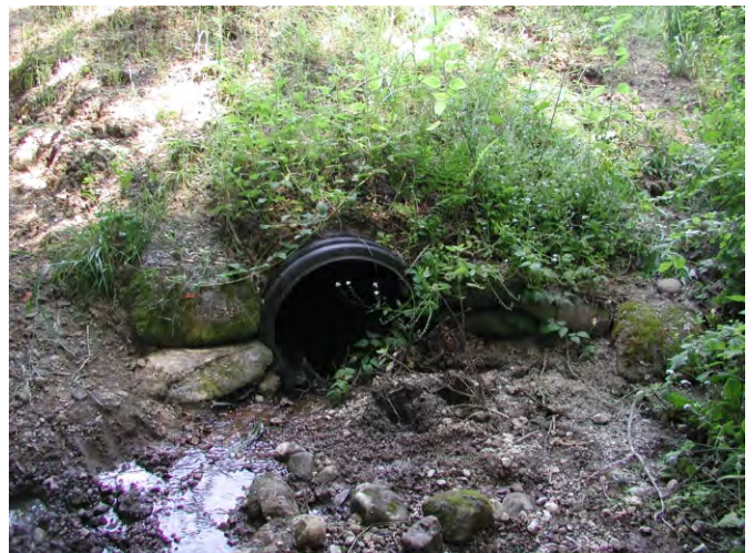
MP 16: 24" culvert inlet. Culvert is undersized and
