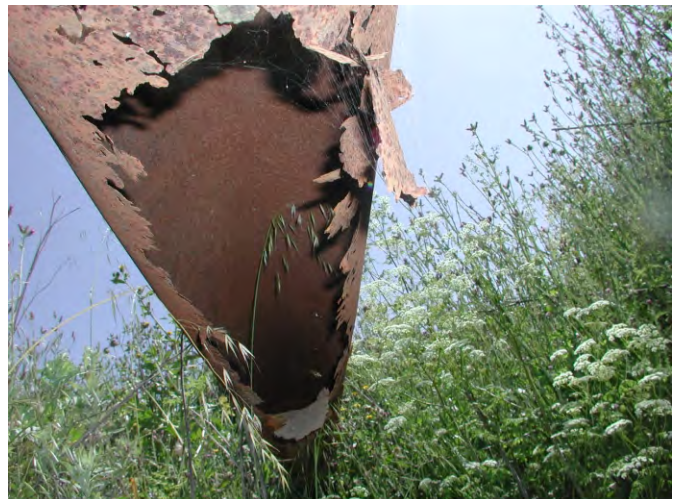
MP 49: Rusted pipe
