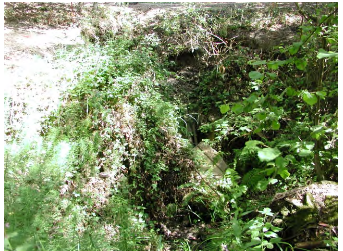
MP 34: Inlet to crossing - note failing concrete headwall
