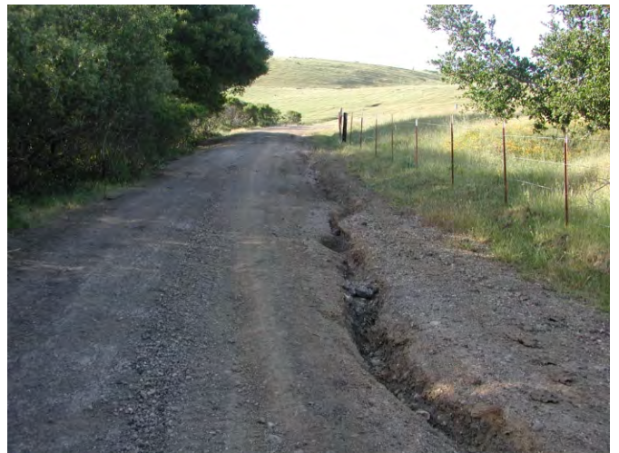
MP 40: Eroding road surface due to concentrated road
