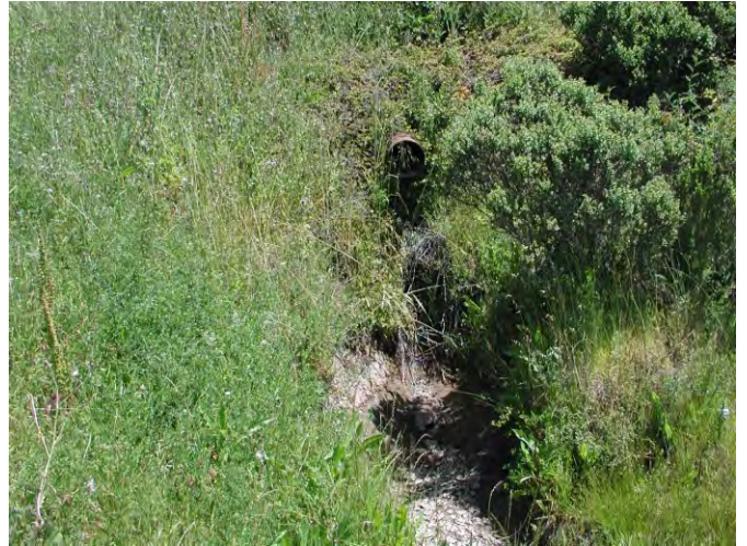
MP 8: Gully at culvert outlet
