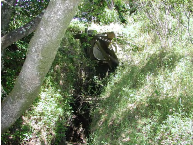
MP 6: Failing wood retaining wall at culvert outlet.
