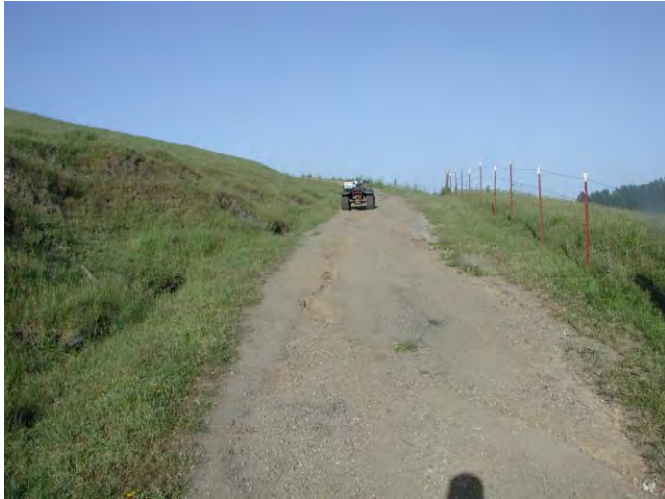
MP 41: Mid portion of long inboard ditch
