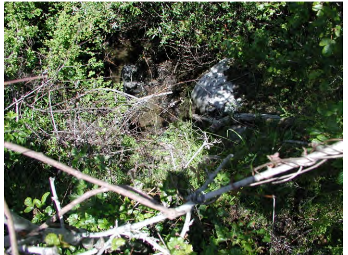
MP 9: Outlet erosion
