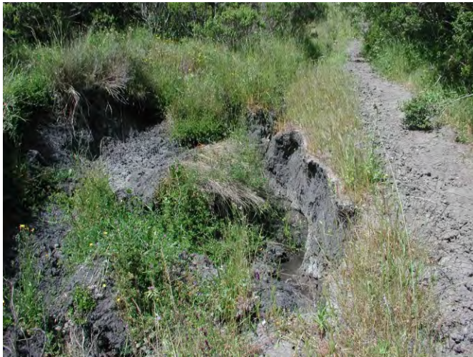
MP 55: Looking up at upper gully.
