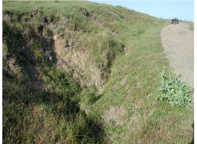
MP 41: Eroding long inboard ditch.
