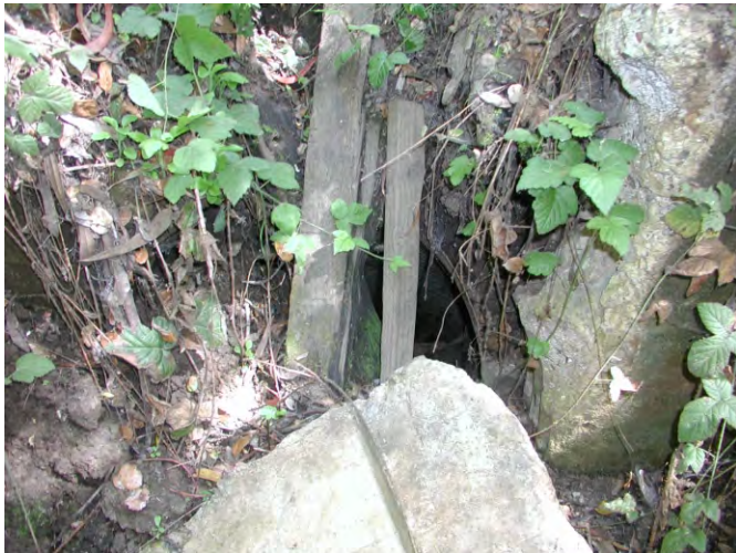
MP 34: Photograph of culvert inlet. Pipe is rusted out
