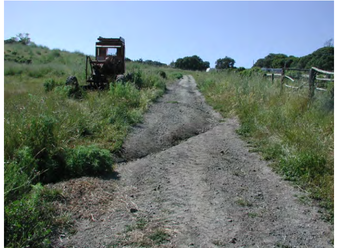
MP 17: Poorly drained rocky road extending up fallline
