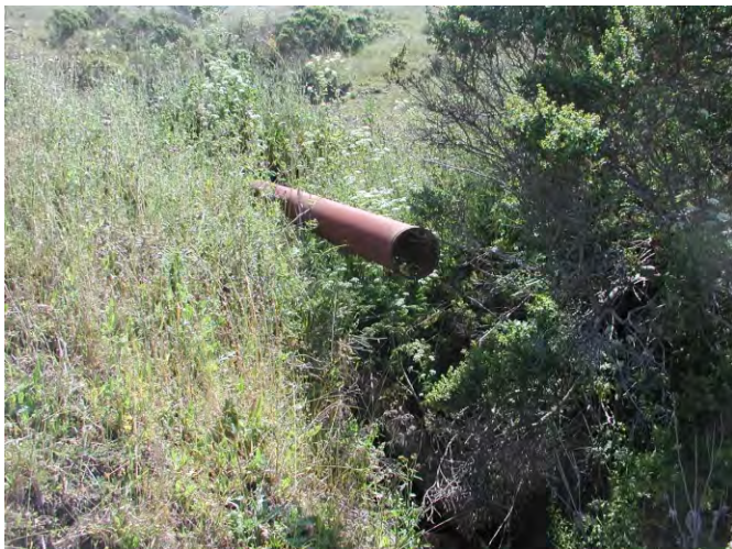
MP 49: Shotgunned culvert outlet
