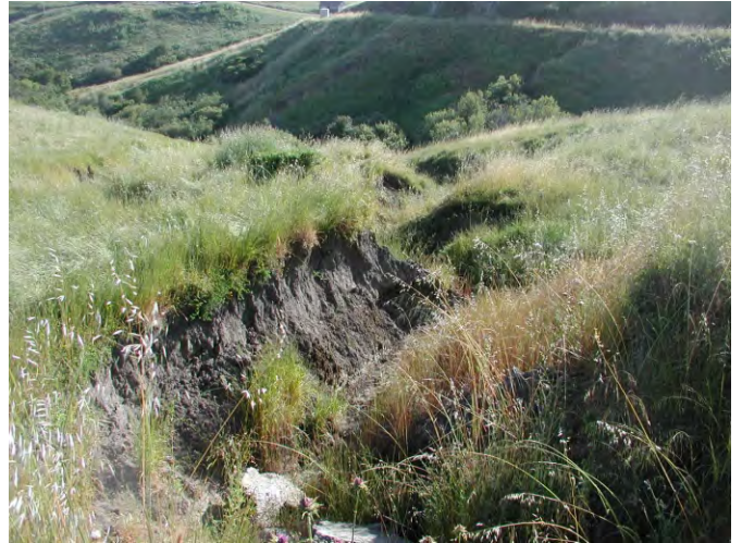
MP 24: Deep gully below ditch relief culvert
