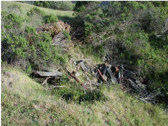
MP 41: Outlet of eroding long inboard ditch
