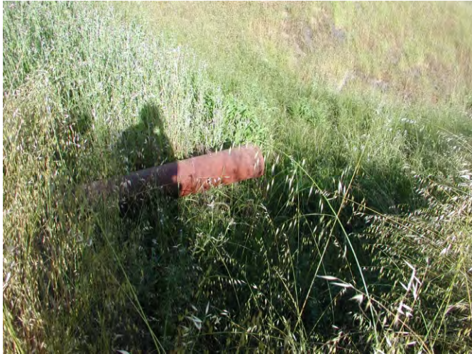
MP 22: Shotgunned culvert outlet
