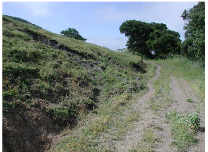
MP 46: Cutbank failure slumped onto road.
