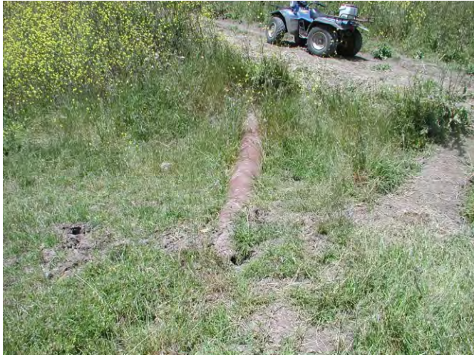
MP 31: Plugged culvert outlet.
