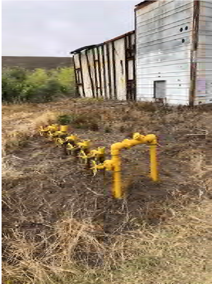
Photo 3. Pipe manifold located next to main access road.
