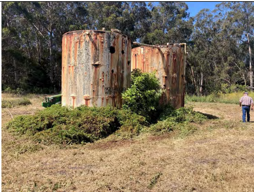
Photo 4. Lower area tanks and access road surrounded by grassland and eucalyptus trees.
